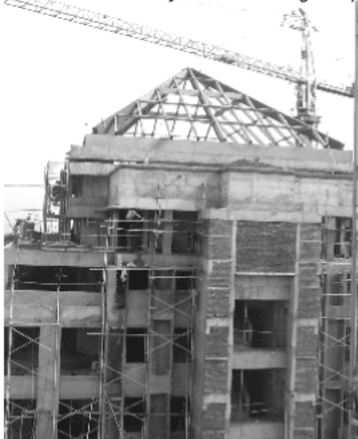
Construction of 40 tonne Prismatic, MS dome having clear height of around 345 feet at ASHFORD - Lower Parel
